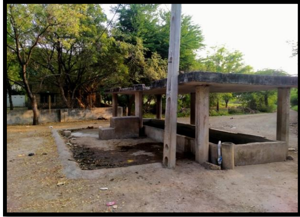
(figure 4.8 ground tank in Katawana)
